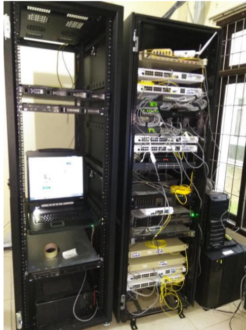
Gambar 3. Ruang Server IAIN Langsa
